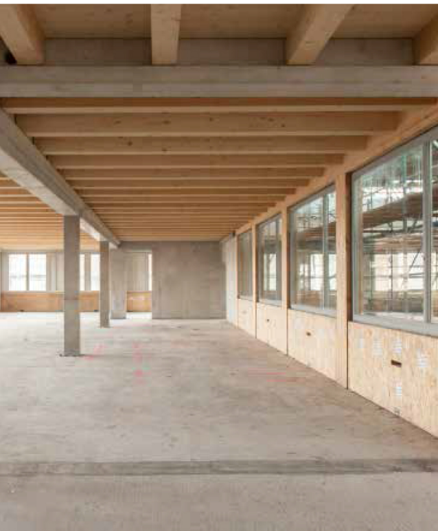
Shell construction of the second floor with a load-bearing structure made of reinforced concrete, timber-concrete composite ceilings and a timber frame façade.
